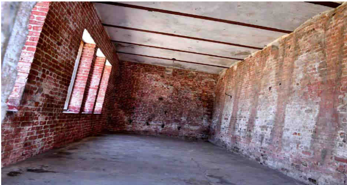
The Interior of the Giddy House Photo Courtesy of the JN Foundation
