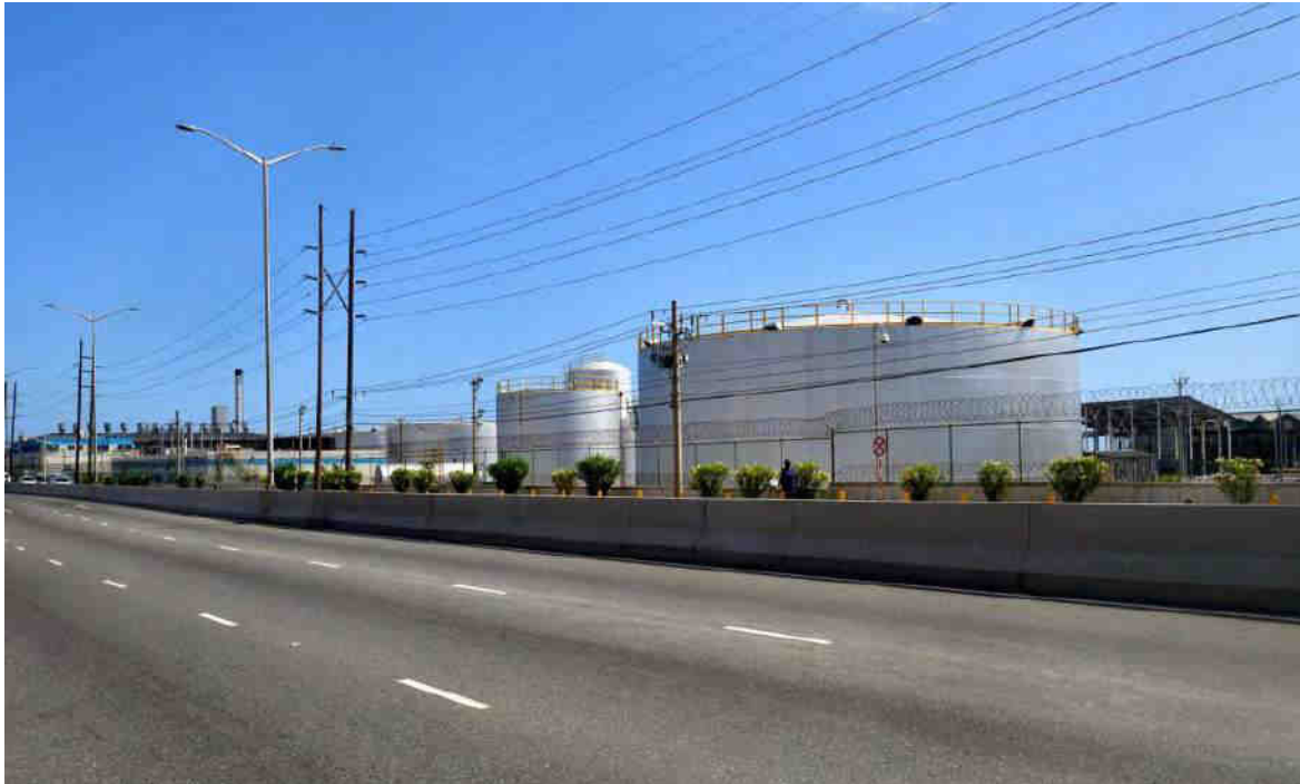
The Esso Refinery now the Petroleum Corporation of Jamaica on Marcus Garvey Drive Photo Courtesy of the JN Foundation
